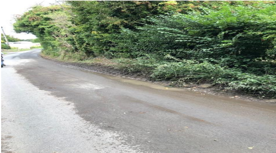
3. Showing the extent of the flooding after a minor rainfall.
