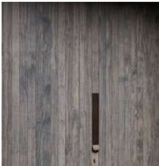
Stained timber cladding
