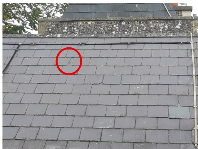
Photograph 7. Broken slate on the southern roof.
