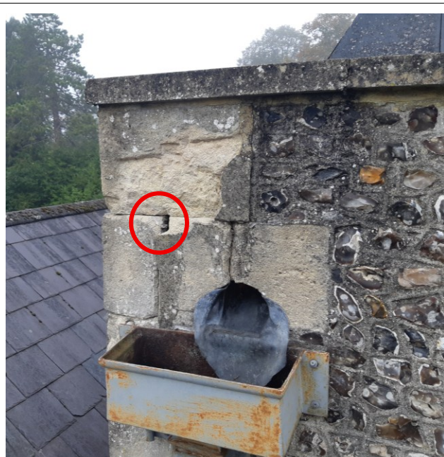
Photograph 5. Crevice above rain drainage hopper on north elevation of the tower.
