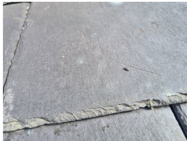
Photograph 4. Bat dropping on slate roof (22 nd July 2025).
