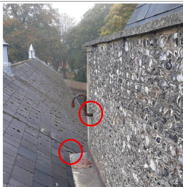
Photograph 6. Pipe in south wall of the tower and broken slate at in the main roof at the southwest corner of the tower wall
