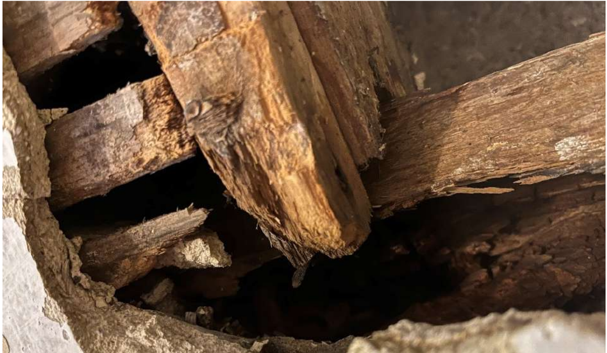
Figure 23 – Evidence of degraded roof timbers due to water ingress
