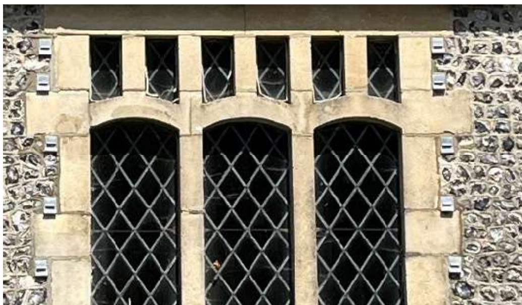
Figure 24 – Example of knapen vent caps installed to other areas of the building
