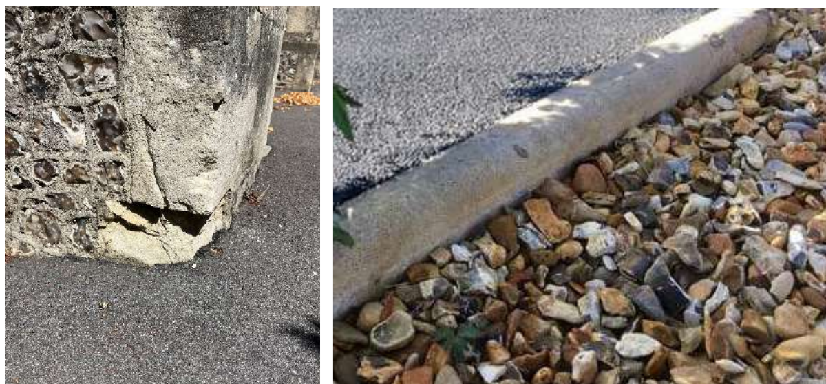
Figure 37 & 38 – Damage caused by impermeable surfaces against building fabric (left), proposed pink kerbing and flint gravel (right)
