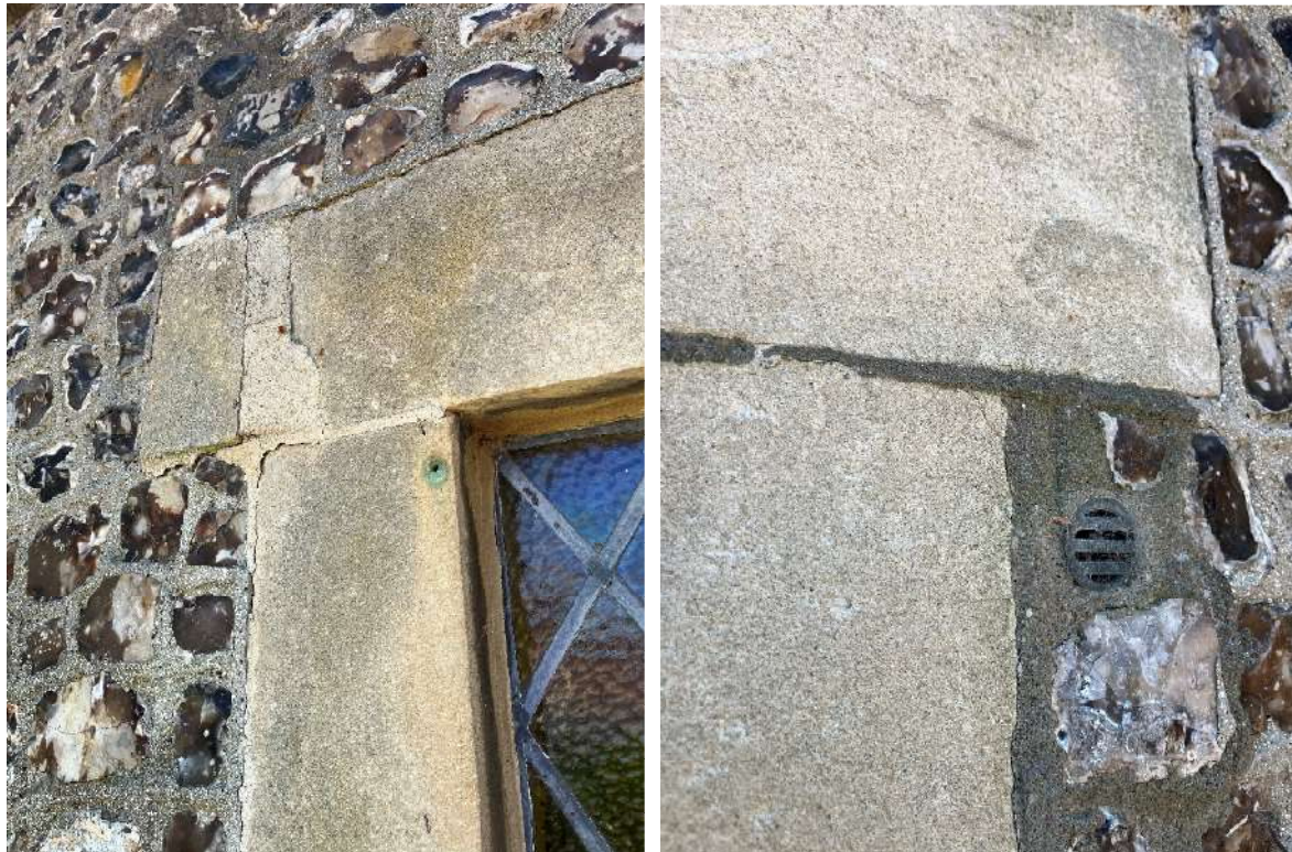
Figure 18 & 19 – Example of poor-quality repairs to stonework (left) and badly matched cement pointing (right)
