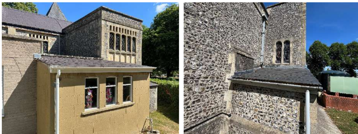
Figure 7 & 8 – Photographs of low pitch vestry roof (left) & store roof (right)
