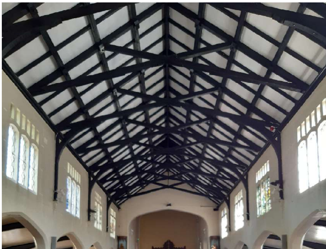
Figure 28 – Asbestos soffit tiles above the scissor trusses to the Nave
