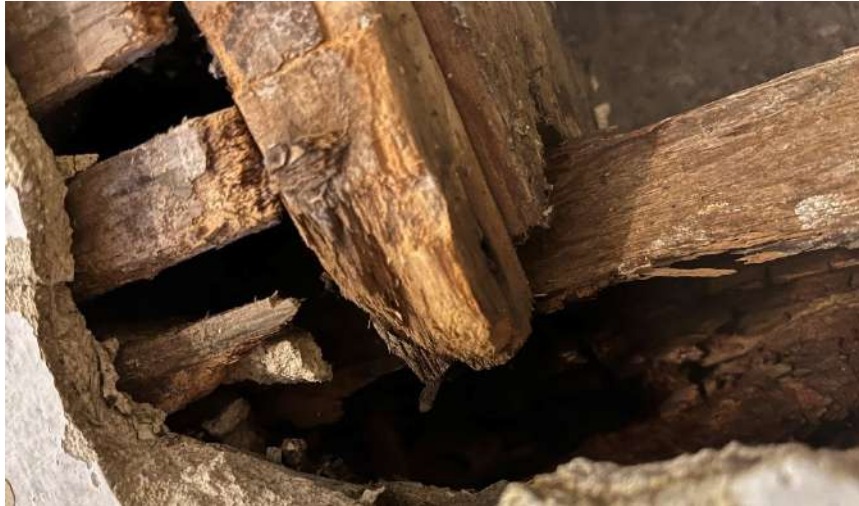
Figure 16 – Evidence of degraded roof timbers due to water ingress
