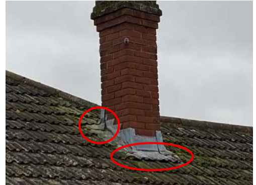
Plate 19: Low condition side porch tiles
