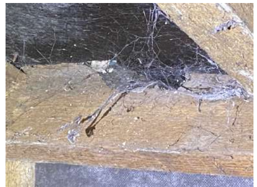
Plate 26: Patched roof felt
