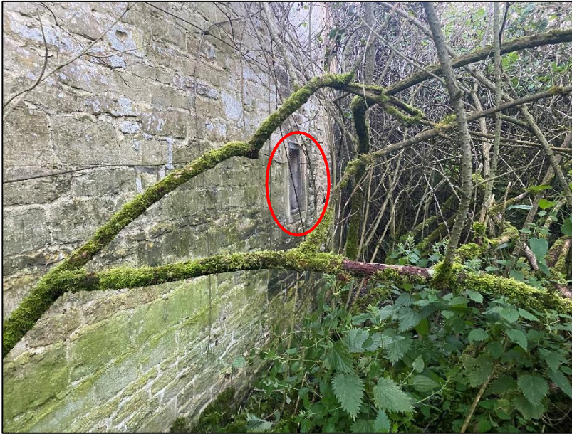
Photograph 7: Broken window on western elevation of Building 3
