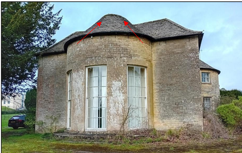
Photograph 6: Gaps under tiles of Building 1
