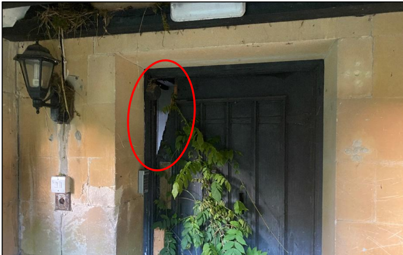
Photograph 5: Gap adjacent Front door of Building 1
