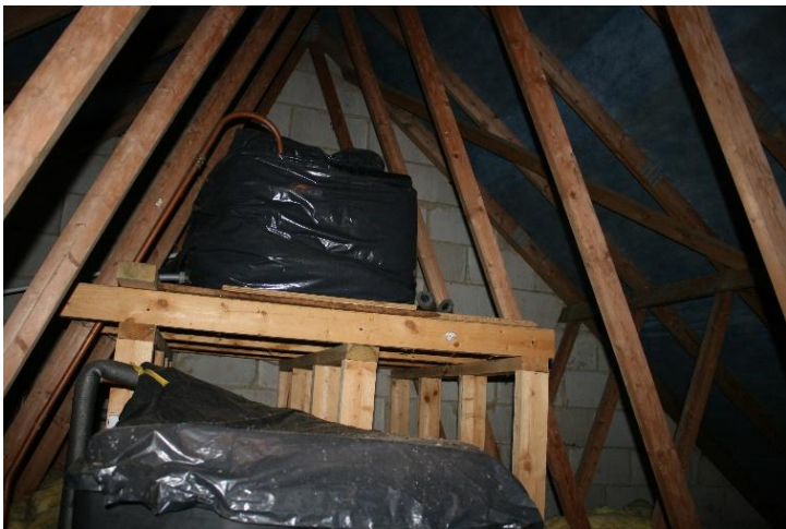
Photo 1: Water tank in the loft void.
