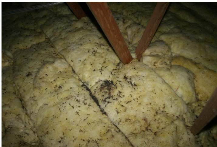
Photo 5: Bat droppings in the loft.
