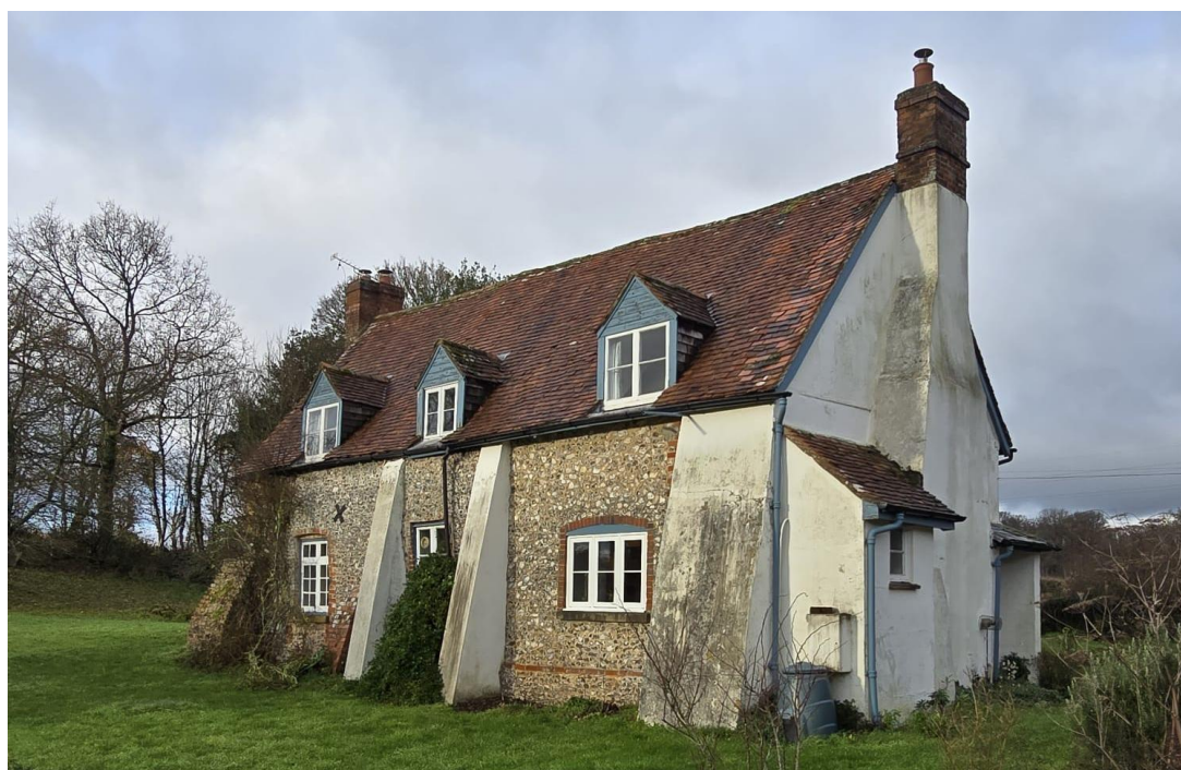
Figure 5 – Rear Elevation of Jolly's Farmhouse prior to roof repair
