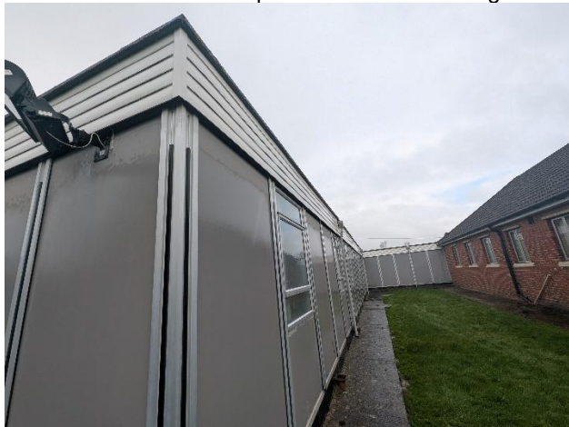
Plate 5: Rotten roof decking/fascia on the roof extension/tank room.
