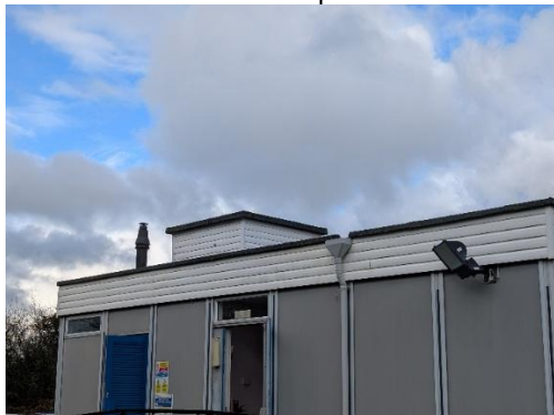
Plate 2: Rotten roof decking/fascia on the roof extension/tank room.
