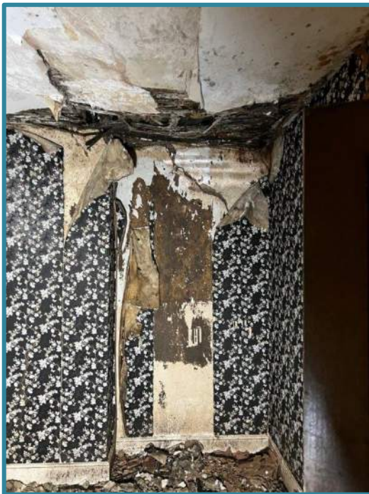
Figure 22 – Plaster fracturing to F.F. landing arch
