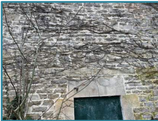
Figure 30 – Fractured lintel NW elevation
