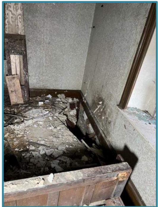
Figure 15 – G.F. Room 4 Failed area of suspended floor
