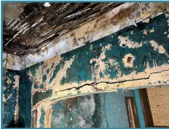
Figure 18 – Plaster fracturing to F.F. landing arch
