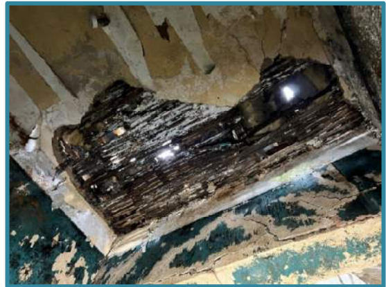
Figure 19 – Daylight visible through central valley soffit
