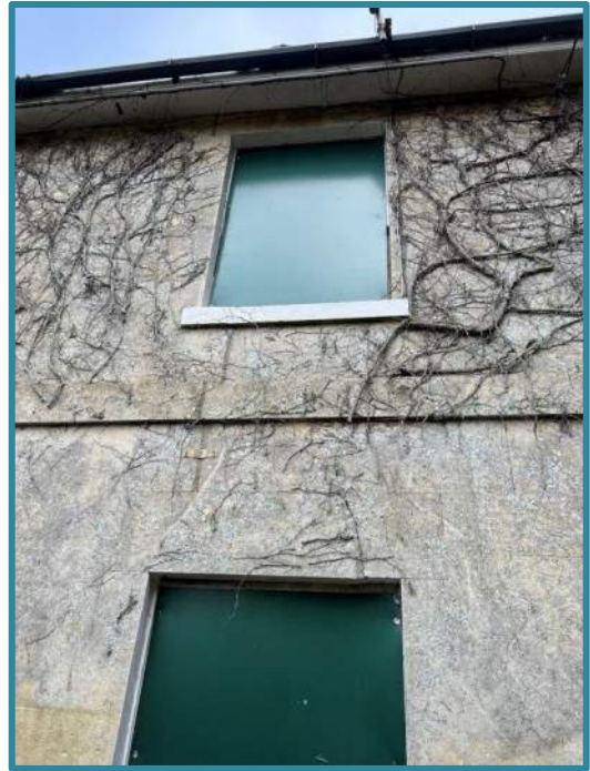
Figure 29 – Fractured lintel SW elevation
