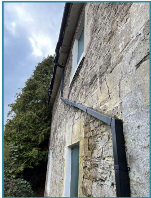
Figure 27 – Slight bulge to southeast elevation
