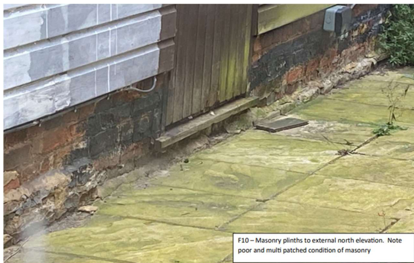
Photograph showing poor condition of masonry plinth to existing outbuilding (taken from GSA report)
