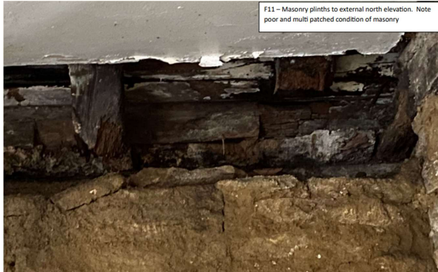
Photograph showing poor condition of masonry within existing outbuilding (taken from GSA report)
