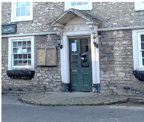
Kerb and uneven paving to main entrance
