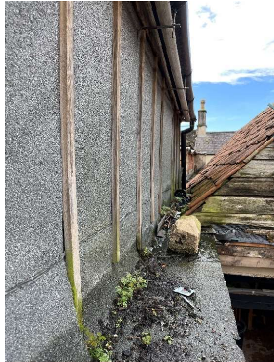
2.6) The side wall of the neighbouring building has bitumen felt secured with timber battens that is in need of a permanent repair.
