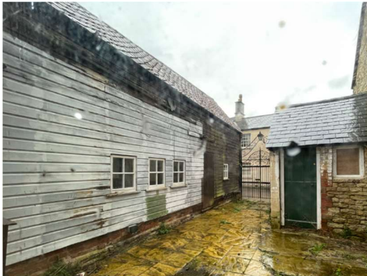
2.11) The timber clad wall facing the courtyard has shiplap cladding, showing signs of degradation and with poorly applied paint finish.
