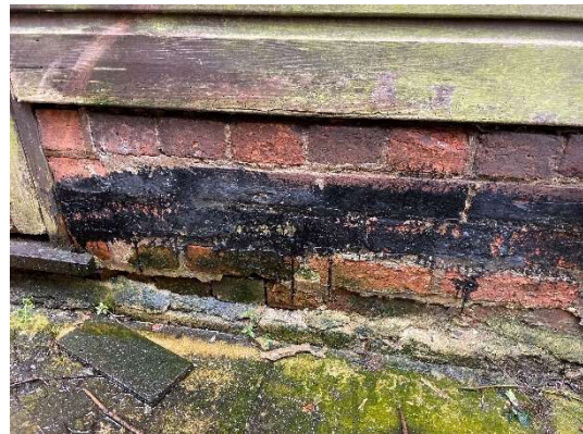
2.8) In places the brickwork facing the courtyard is spalling and has been painted with what appears to be bituminous paint.
