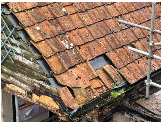
2.3) Detail photo showing the degraded pantiles, modern roofing felt and PVC guttering. The degraded timber cladding is also visible.
