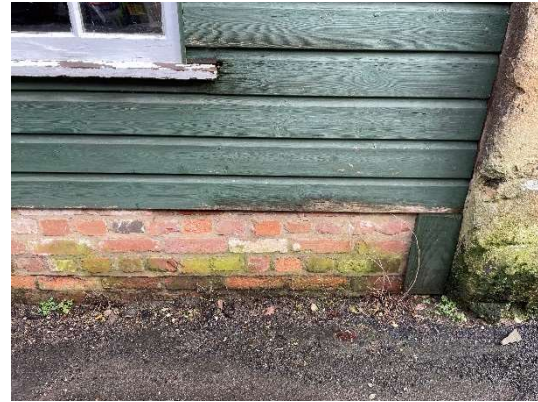
2.10) Window frames and cladding showing signs of degradation.
