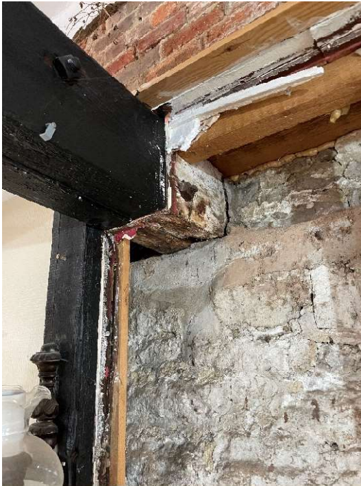
3.9) The South wall has been lined with plasterboard on softwood framing. A section of plasterboard has been removed to expose the party wall, this reveals the floor joists bearing onto the stone wall. Joist ends have rotted in the past and these have been repaired with new timber supports.
