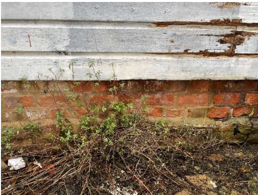
2.7) The brick plinth wall is visible on the courtyard facing elevation, there is a course of stonework at the base with brickwork above laid in English bond. Timber cladding shows signs of degradation and poorly applied white paint.
