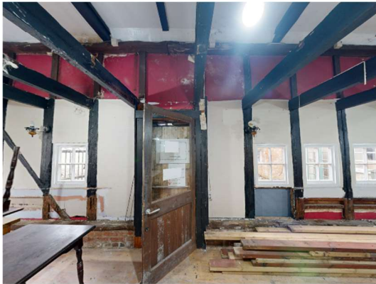
3.3) Fixed casement window and glazed door. Effects of water ingress at eaves evident on upper part of the wall.
