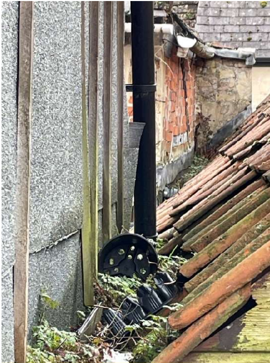
2.5) The valley gutter above the party wall is blocked and appears to be formed from loose bitumen felt. The guttering to the neighbouring building is also in need of attention.
