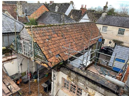
2.2) Roof and East facing gable, illustrates poor condition of pantile roof. The gable is clad with shiplap cladding with a modern casement window. Timber cladding and window frame are in poor condition.
