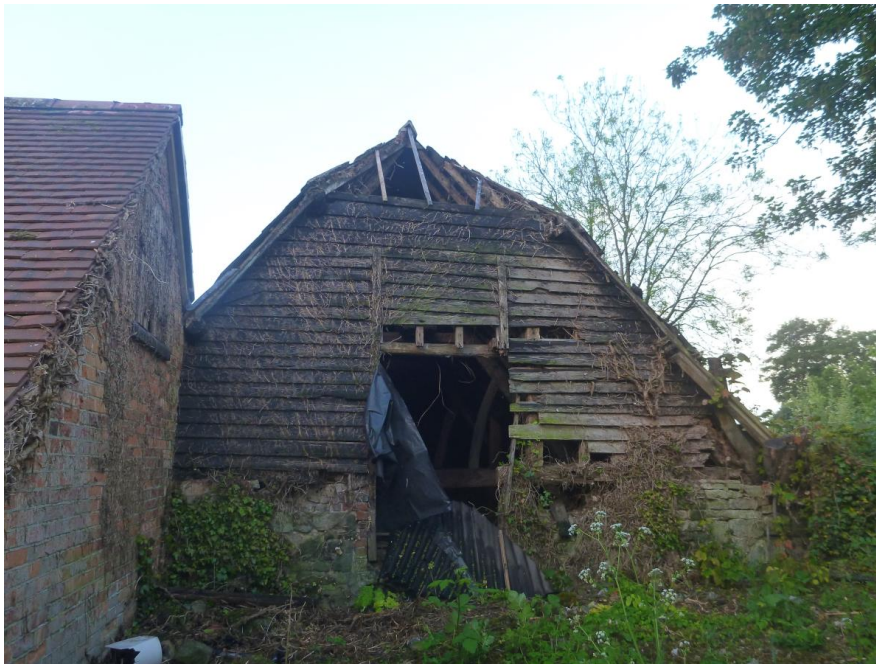
Fig 6: The north face of Barn A is particularly exposed to the elements.
