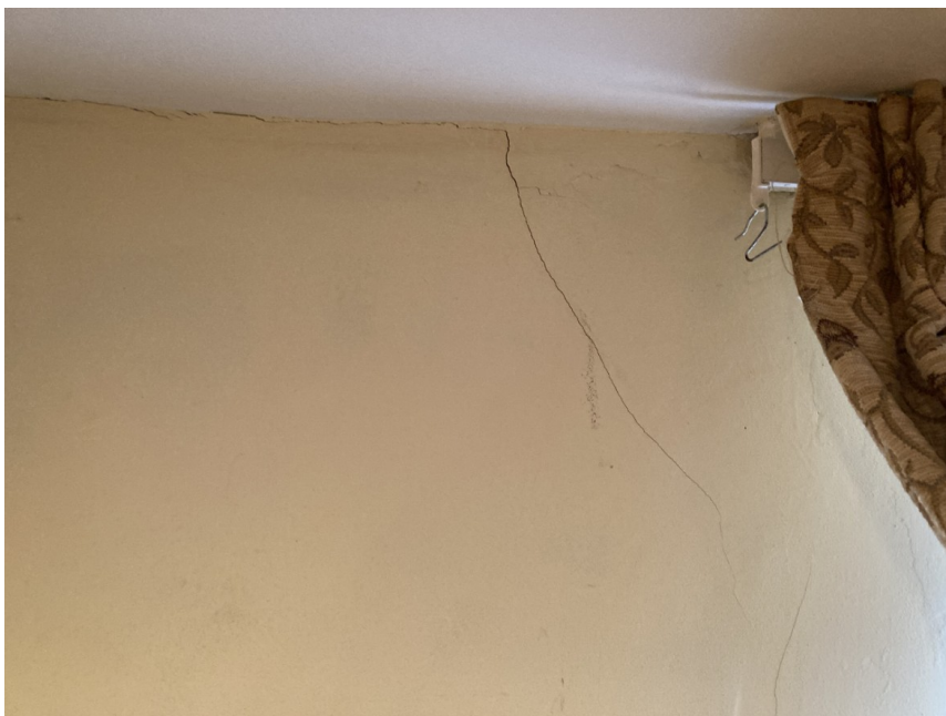
3. Diagonal crack on the internal face of the external front wall
