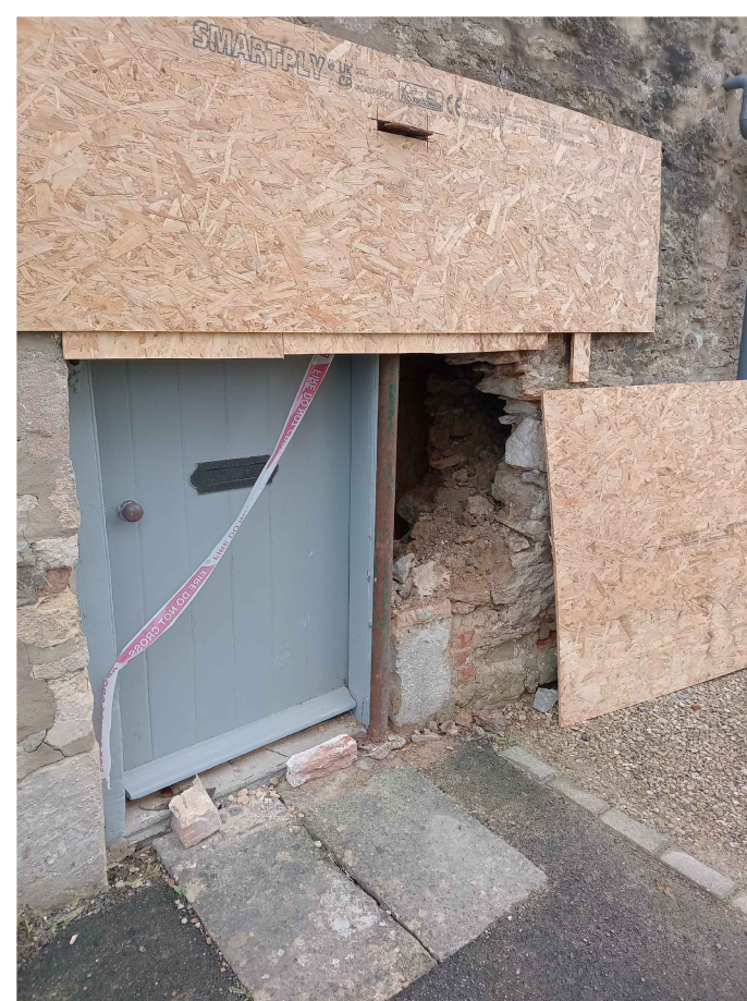
Photo 2: View of the damage caused externally
