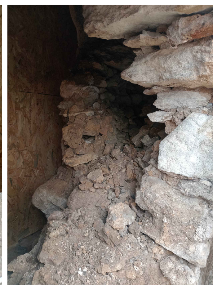
Photo 5: Close up of the damage to masonry
