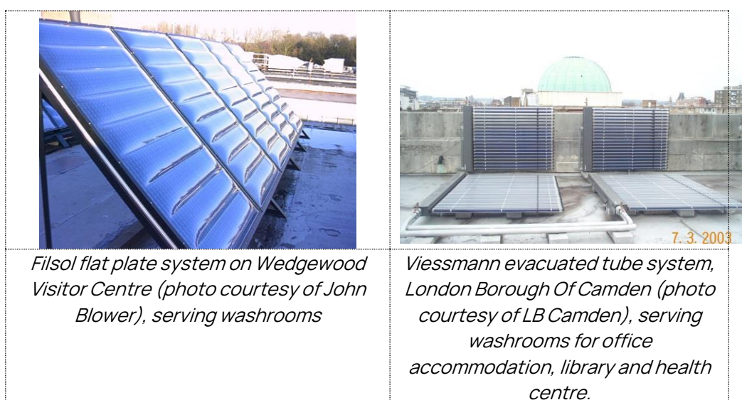
Figure 3 - Typical Solar Thermal Collectors
