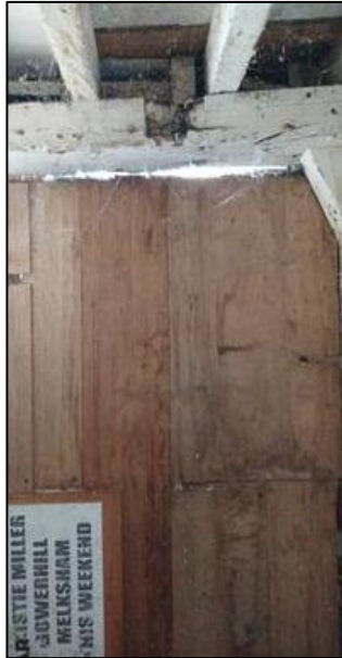
Photo 5 Gap above doorway
