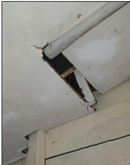
Photo 7 Hole in ceiling
