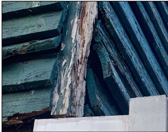
Photo 3 Gaps under wooden panelling
