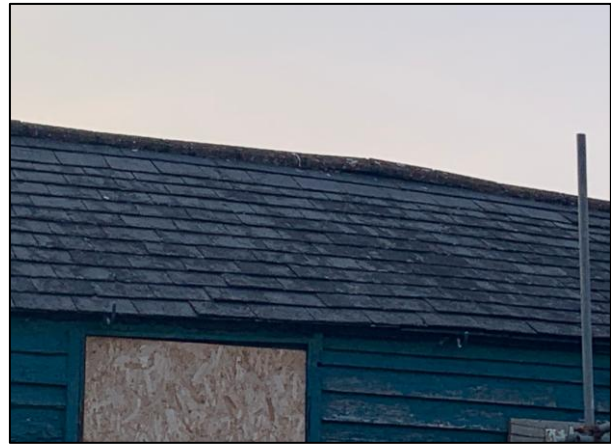
Photo 4 Lifted ridge tiles on eastern end of building
