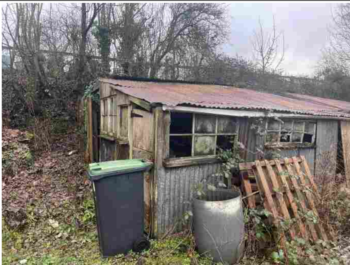
PLATE 6 – Another dilapidated shed on the eastern boundary
