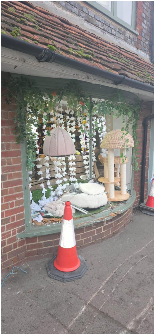
Shopfront entrance door (showing wood and glass has been damaged):
