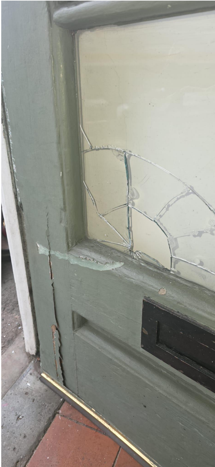
Shopfront lean-to roof (showing damage and movement to some of the roof tiles, movement of leadwork and damage from impact to the guttering/downpipe):
