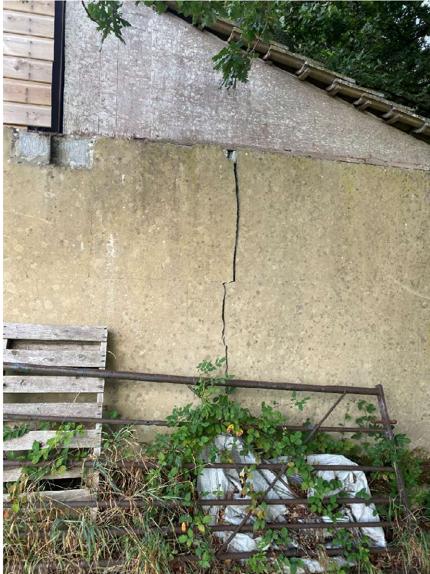
Figure 1.12 – Vertical crack on gable elevation
