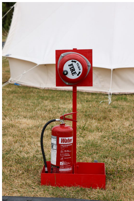
An example of a fire call point that are site around the camp site
