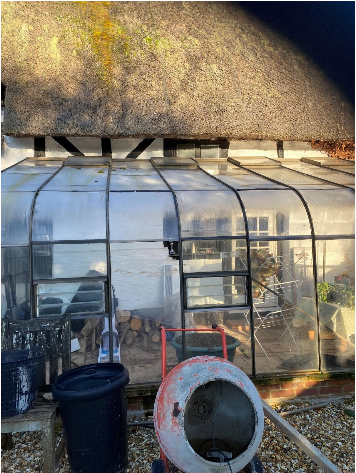
PHOTO 6 – REAR ELEVATION SHOWING HOW THE EXISTING CONSERVATORY DISSECTS THE Ff WINDOW
