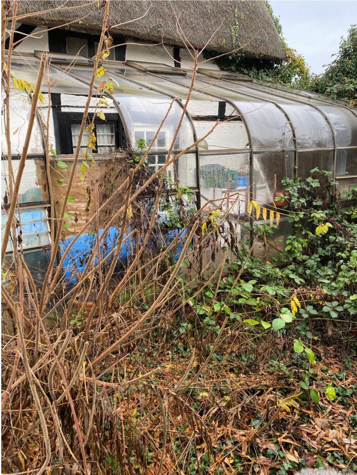
PHOTO 3 – REAR ELEVATION SHOWING HOW THE EXISTING CONSERVATORY CLASHES WITH THE FF WINDOW
