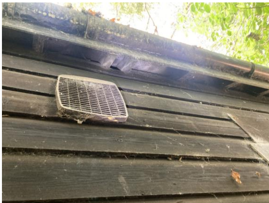
Figure 17 - Gaps in the soffit.
