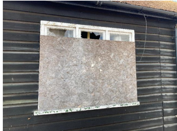
Figure 16 – Scott's Gym, broken window.
