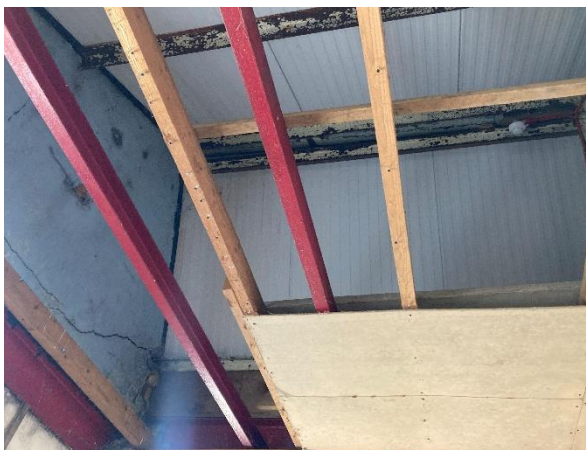
Figure 8 - Loft space of Block D. Large parts of the ceiling of the top floor of Block D were open giving access to the loft space.
