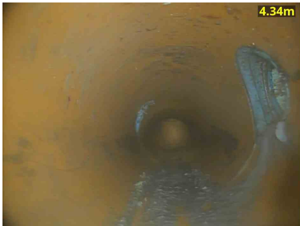
3, 00:00:39, 4.34 m Connection other than junction at 3 o'clock, 40mm dia
