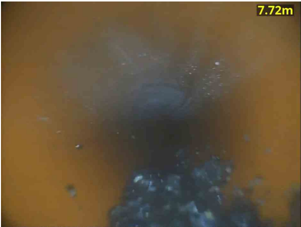
2, 00:06:48, 7.72 m Settled deposits, coarse, 10% cross-sectional area loss
