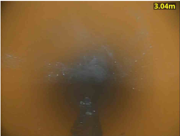
1, 00:07:22, 3.04 m Settled deposits, coarse, 5% cross-sectional area loss
