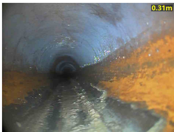
2, 00:00:14, 0.31 m Settled deposits, hard or compacted, 5% cross-sectional area loss, start, Scale
