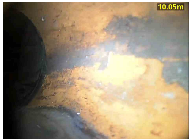
4, 00:01:21, 10.05 m Settled deposits, hard or compacted, 5% cross-sectional area loss, finish, Scale
