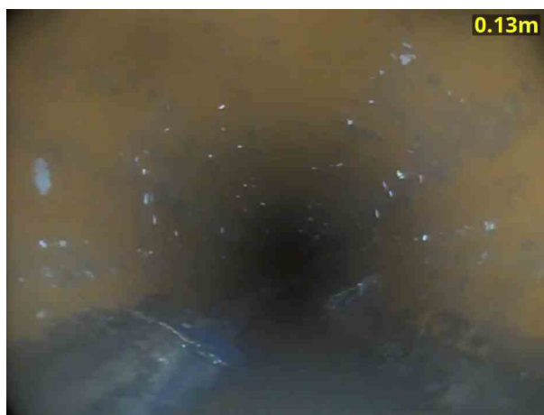
2, 00:00:12, 0.13 m Settled deposits, hard or compacted at joint, 10% cross-sectional area loss, start, Scale
