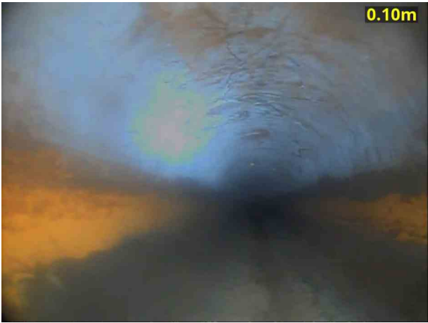
2, 00:00:12, 0.10 m Settled deposits, hard or compacted, 5% cross-sectional area loss, start
