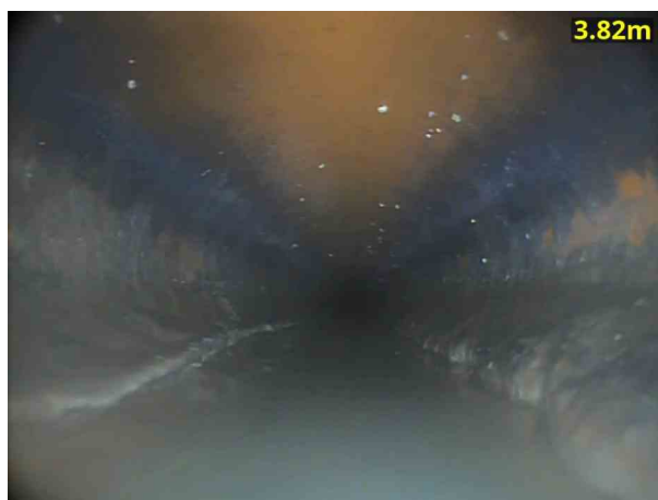
4, 00:00:39, 3.82 m Settled deposits, hard or compacted, 15% cross-sectional area loss
