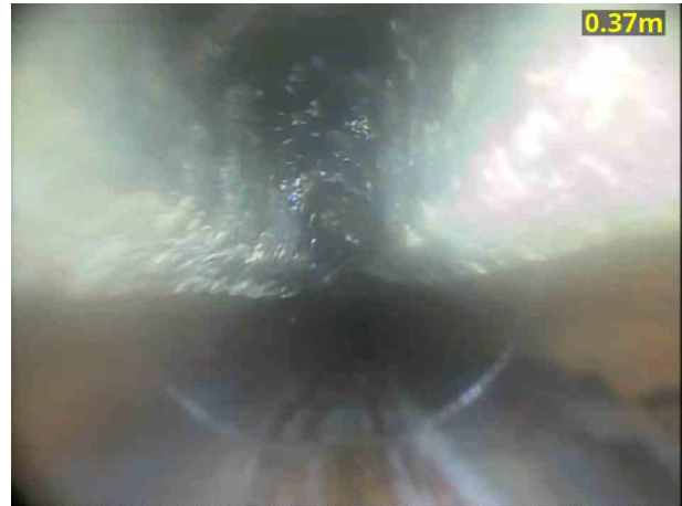
2, 00:00:15, 0.37 m Attached deposits, encrustation from 9 o'clock to 3 o'clock, 25% cross-sectional area loss, start
