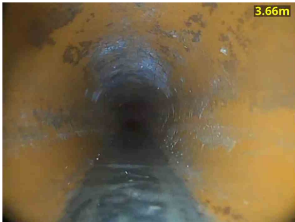
3, 00:00:34, 3.66 m Settled deposits, hard or compacted, 10% cross-sectional area loss, Scale
