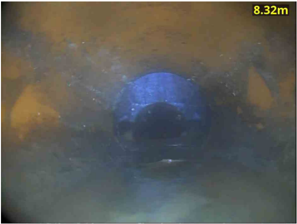
7, 00:01:24, 8.32 m Settled deposits, hard or compacted at joint, 10% cross-sectional area loss, finish, Scale
