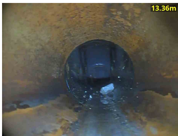
4, 00:01:43, 13.36 m Settled deposits, hard or compacted, 5% cross-sectional area loss, finish, Scale
