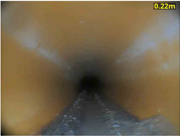
2, 00:00:13, 0.22 m Settled deposits, hard or compacted, 5% cross-sectional area loss, start
