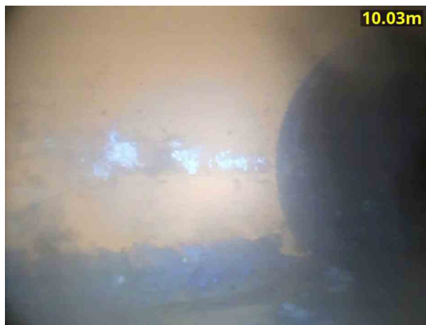
6, 00:01:30, 10.03 m Settled deposits, hard or compacted, 5% cross-sectional area loss, finish, Scale
