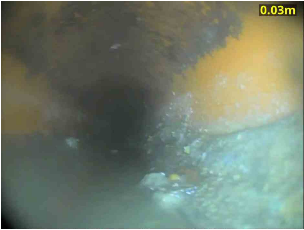
2, 00:00:14, 0.03 m Settled deposits, hard or compacted, 5% cross-sectional area loss, start, Scale
