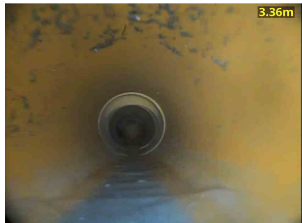
4, 00:00:58, 3.36 m Settled deposits, hard or compacted, 5% cross-sectional area loss, finish, Scale
