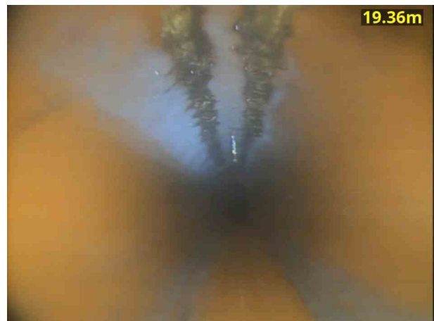
4, 00:02:08, 19.36 m Attached deposits, encrustation at 12 o'clock, 5% cross-sectional area loss, finish
