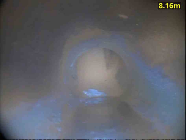
3, 00:01:19, 8.16 m Settled deposits, hard or compacted, 5% cross-sectional area loss, finish, Scale
