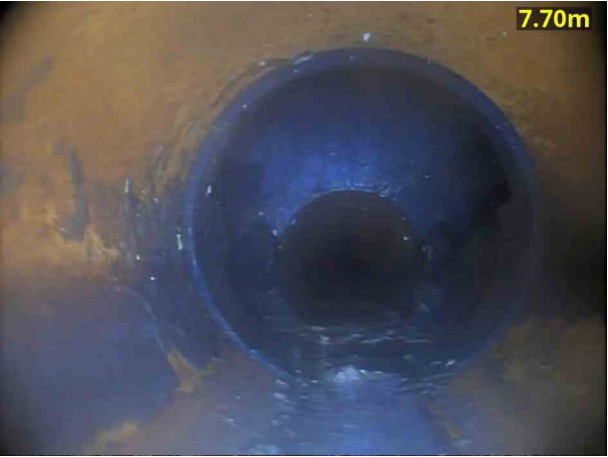
3, 00:01:05, 7.70 m Settled deposits, hard or compacted, 5% cross-sectional area loss, finish, Scale
