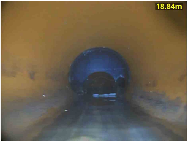
10, 00:02:44, 18.84 m Settled deposits, hard or compacted, 5% cross-sectional area loss, finish, Scale
