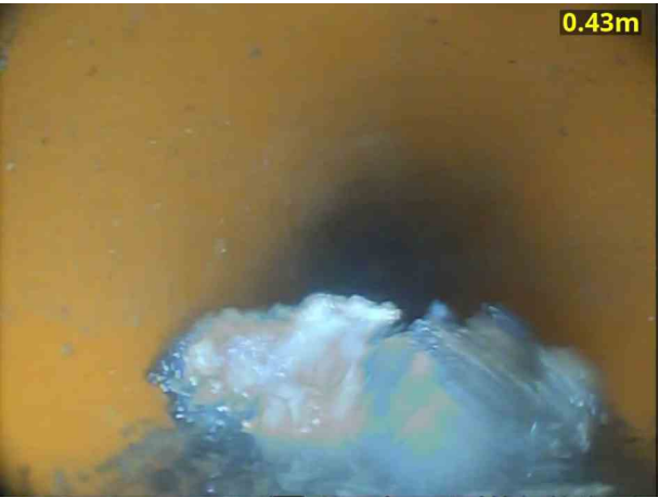
3, 00:00:23, 0.43 m Settled deposits, coarse, 25% cross-sectional area loss
