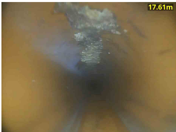
3, 00:01:57, 17.61 m Attached deposits, encrustation at 12 o'clock, 5% cross-sectional area loss, start
