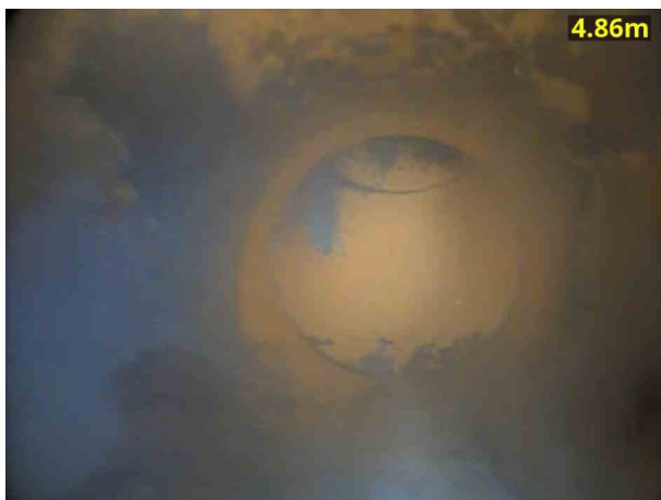
5, 00:00:46, 4.86 m Settled deposits, hard or compacted, 5% cross-sectional area loss, finish, Scale
