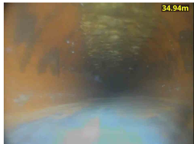
6, 00:04:05, 34.94 m Attached deposits, grease from 10 o'clock to 2 o'clock, 10% cross-sectional area loss, start
