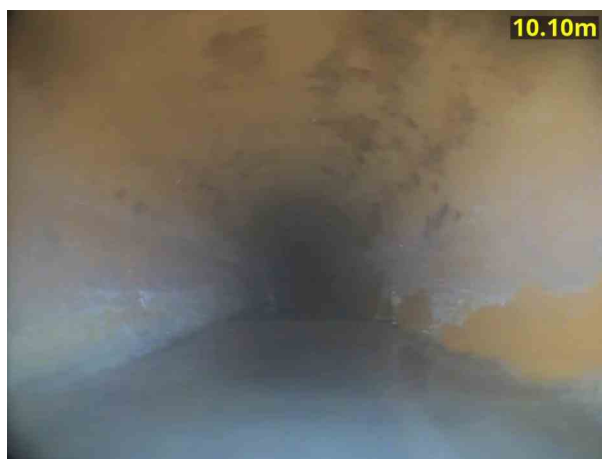
4, 00:01:17, 10.10 m Settled deposits, hard or compacted, 5% cross-sectional area loss, finish
