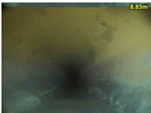
3, 00:01:06, 8.83 m Settled deposits, hard or compacted, 5% cross-sectional area loss, start
