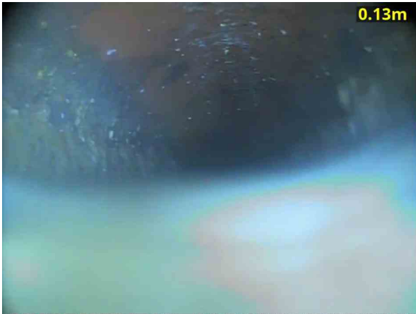
1, 00:01:43, 0.13 m Settled deposits, hard or compacted, 10% cross-sectional area loss, start, Scale
