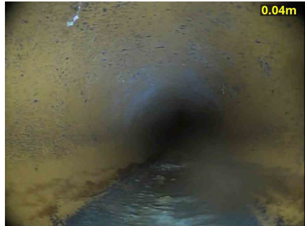
2, 00:00:17, 0.04 m Settled deposits, hard or compacted, 5% cross-sectional area loss, start, Scale
