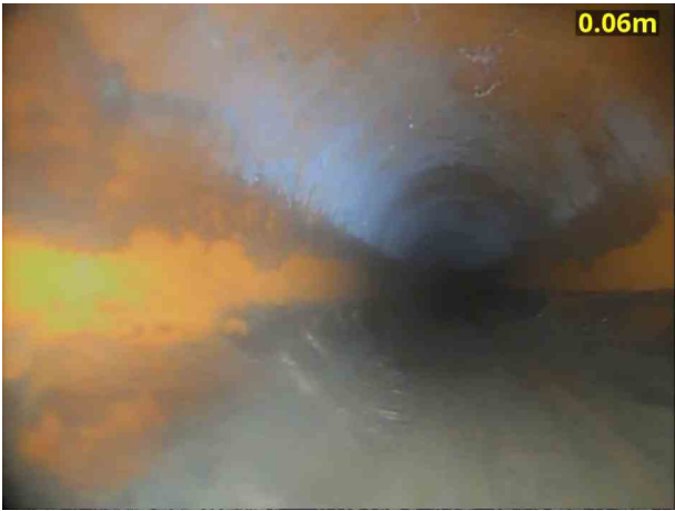
2, 00:00:12, 0.06 m Settled deposits, hard or compacted, 5% cross-sectional area loss, start, Scale
