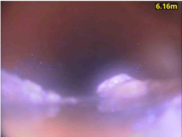
7, 00:01:14, 6.16 m Settled deposits, fine, 20% cross-sectional area loss
