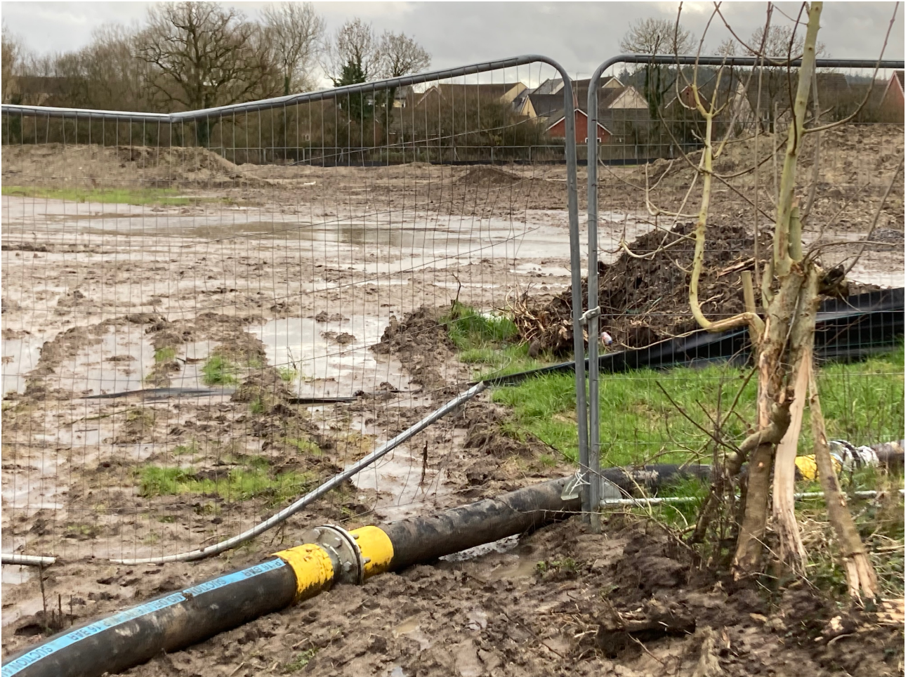
Above: Part of the piping to remove flood water from Jubilee Gardens.
