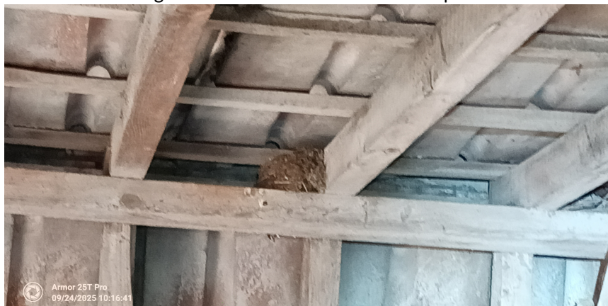
Photo 20. Showing swallow nest on roof timber of open fronted section Cart Shed
