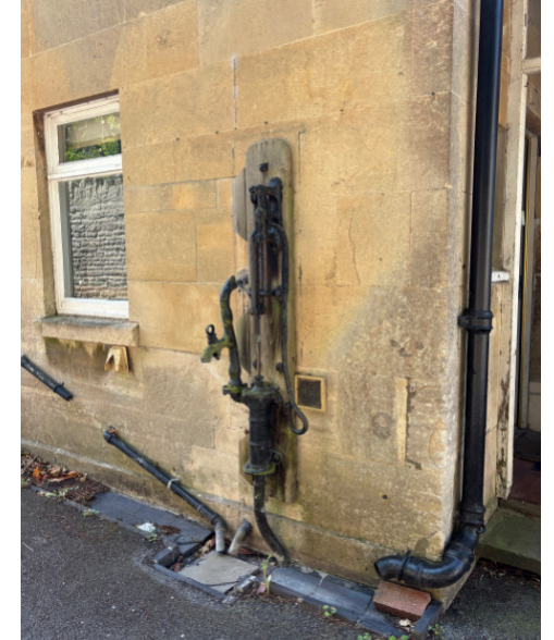
External water pump (north elevation) - to be retained.
