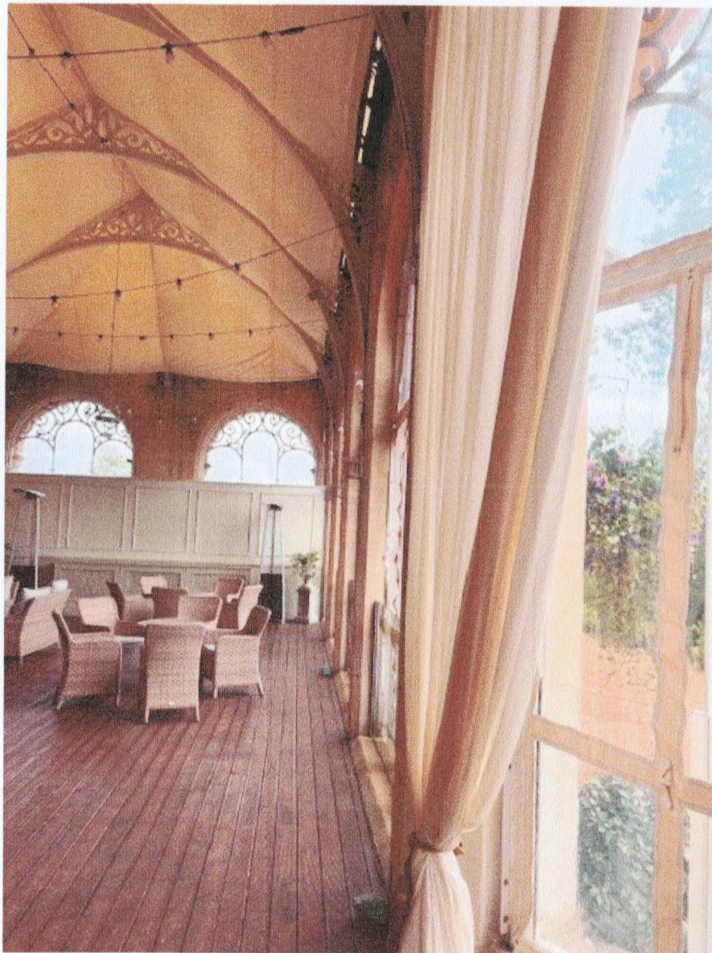
PLATE 02 -- LEANING SOUTHERN ELEVATION WALL
