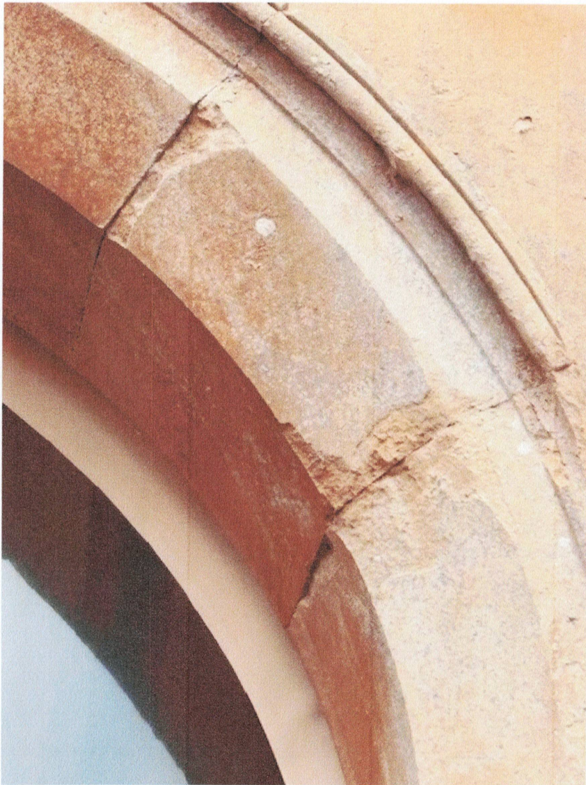
PLATE 03 -- MASONRY DAMAGE IN SOUTHERN WALL ARCH
