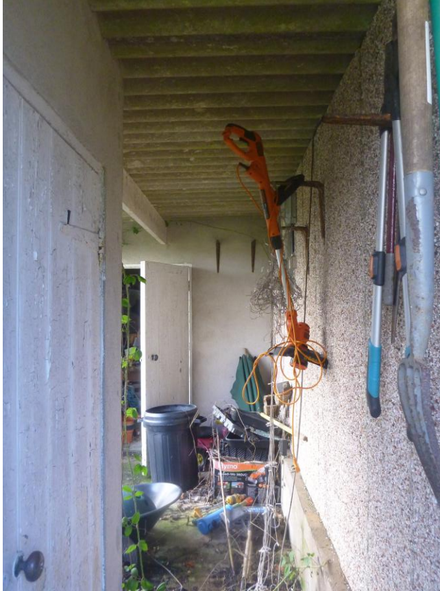
Fig 5: There is an open alcove on the northern face of the garage.
