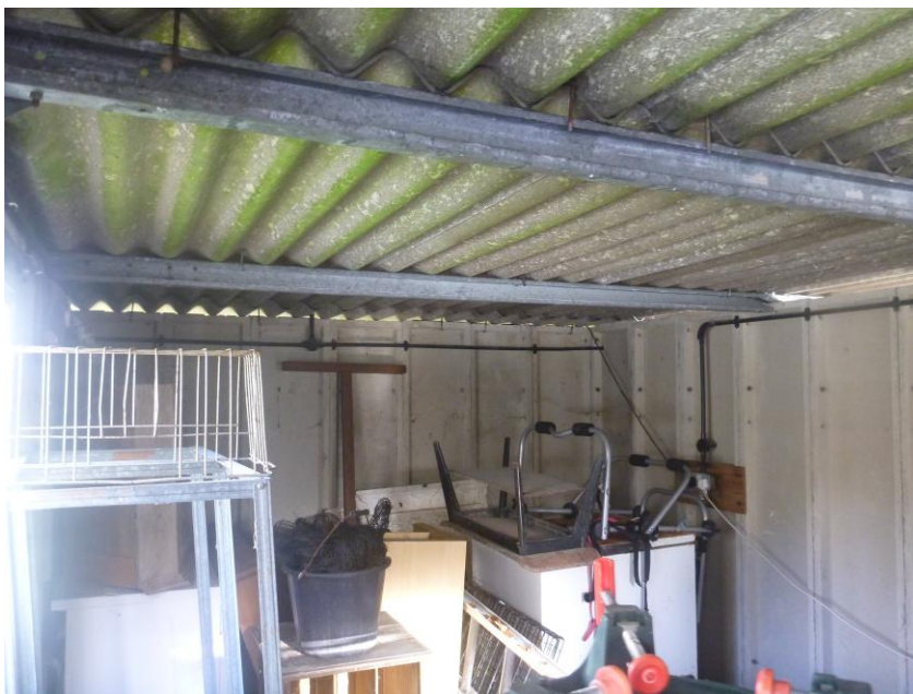
Fig 4: All internal areas of the garage are disturbed by daylight.
