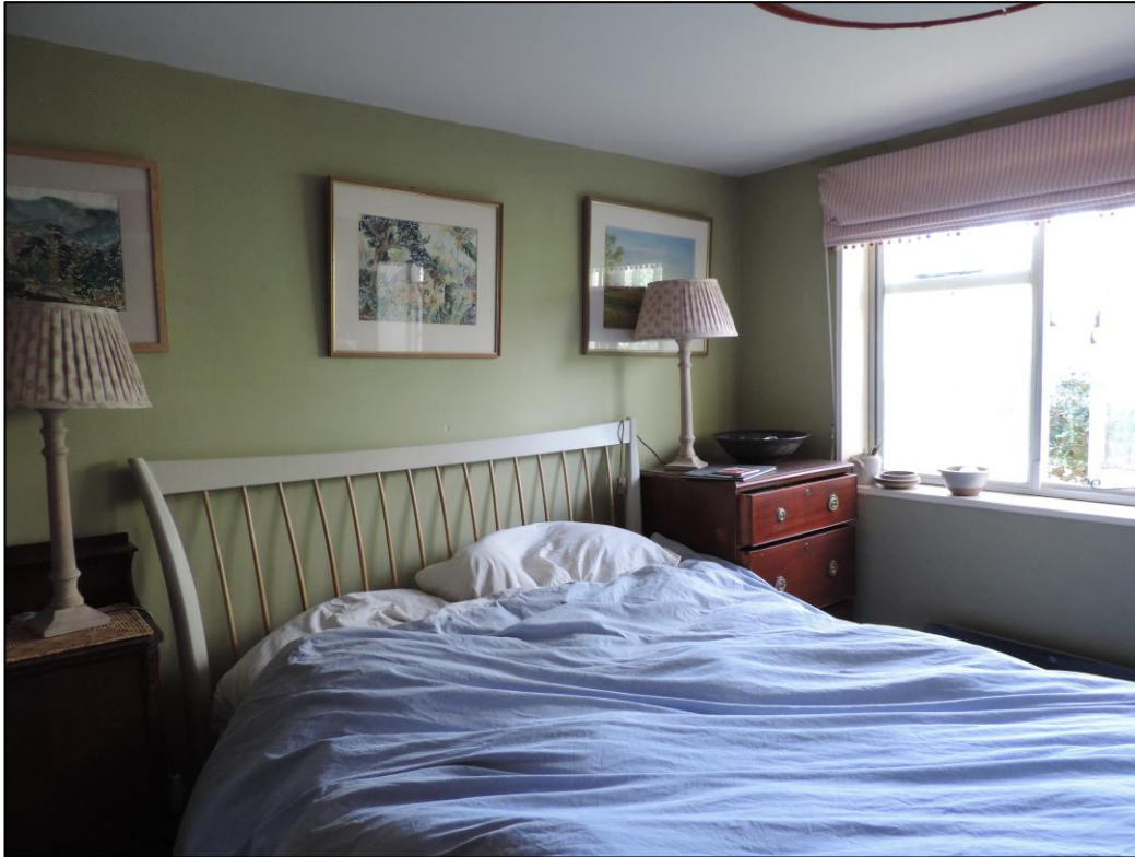
Photo 7 The low ceiling within Bedroom 1 adds to the overall cramped feeling of this room within the 1970s extension.
