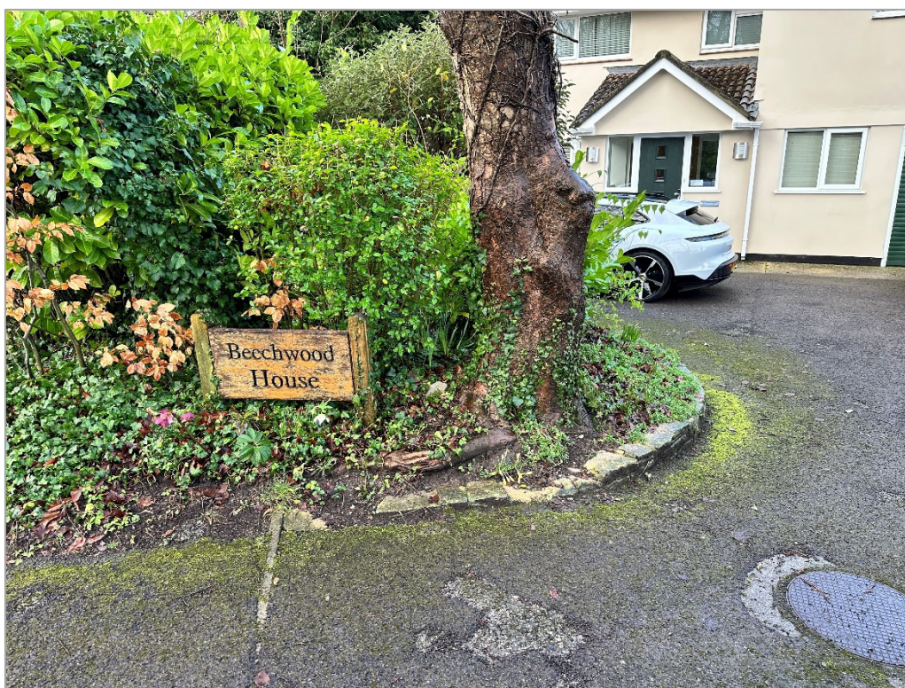
Figure 2: T4 with a surface root that has defected away from the stone wall and tarmac driveway.
