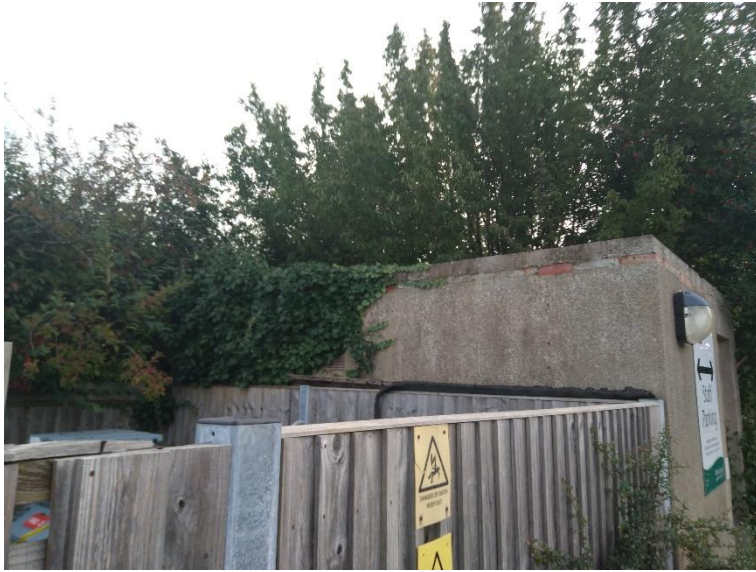
Photograph 2.1: Electrical substation within the site boundary
