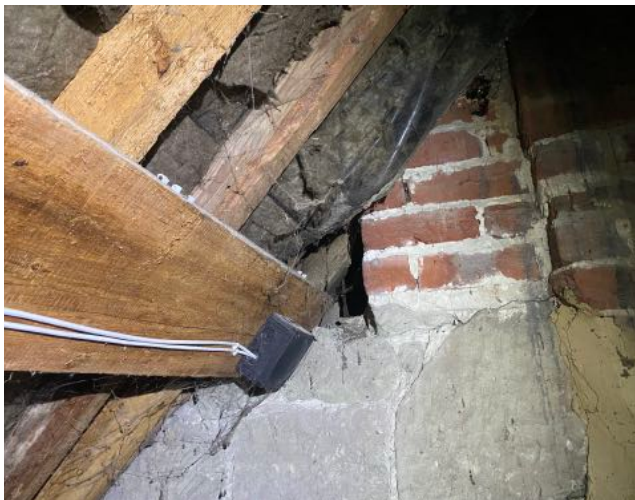
Image 22: Gap between eastern chimney and roof of L2.
