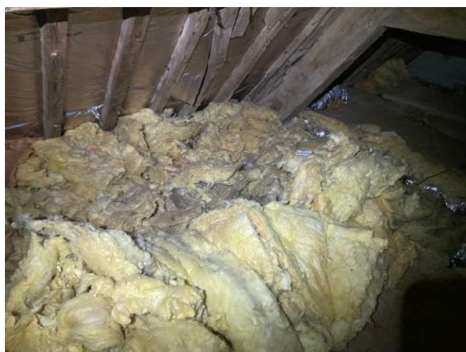
Image 21: Pile of old insulation towards the southern aspect of L1 where droppings were found.
