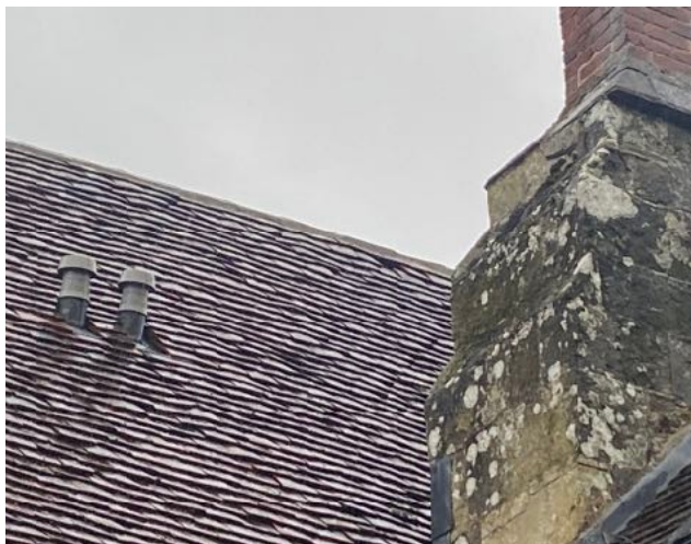
Image 18: Missing tile on western aspect of B1.
