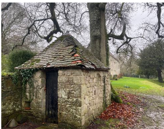
Image 27: South aspect of B4 with multiple missing / slipped roof tiles.
