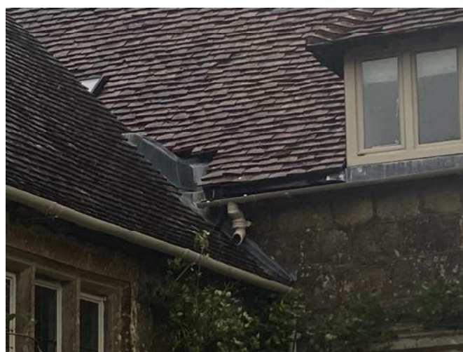
Image 19: Raised roof tiles on lower southwest aspect of B1.
