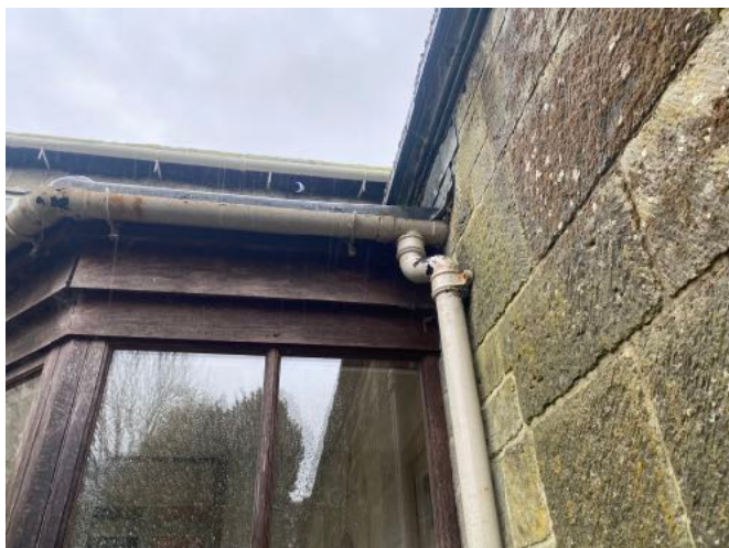
Image 17: Crevice under lead flashing of small extension connection B2 to the underground pool.
