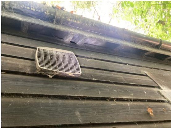
Figure 17 - Gaps in the soffit.
