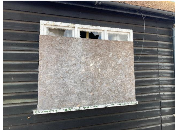
Figure 16 – Scott's Gym, broken window.
