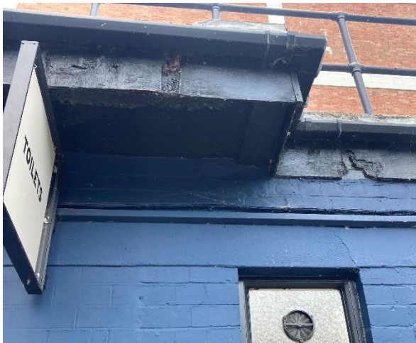
Figure 13 - Rotten woodwork on the toilet block on the south side of the main building.
