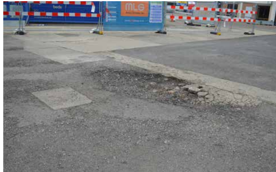
1 - Degraded tarmac and concrete surface
