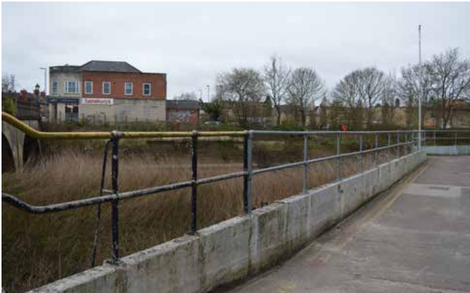
5 - Mixture of recent key clamp and older railings
