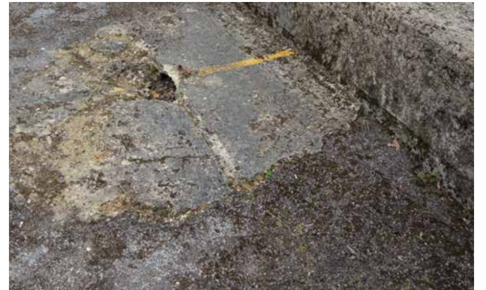
2 - Degraded concrete surface and historic foundation
