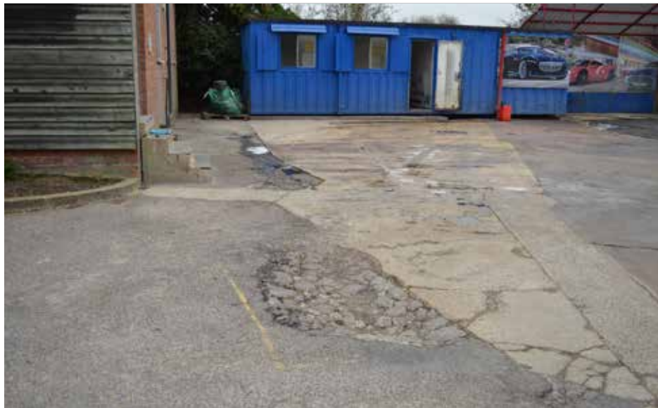
3 - Subsided tarmac and fractured concrete surface
