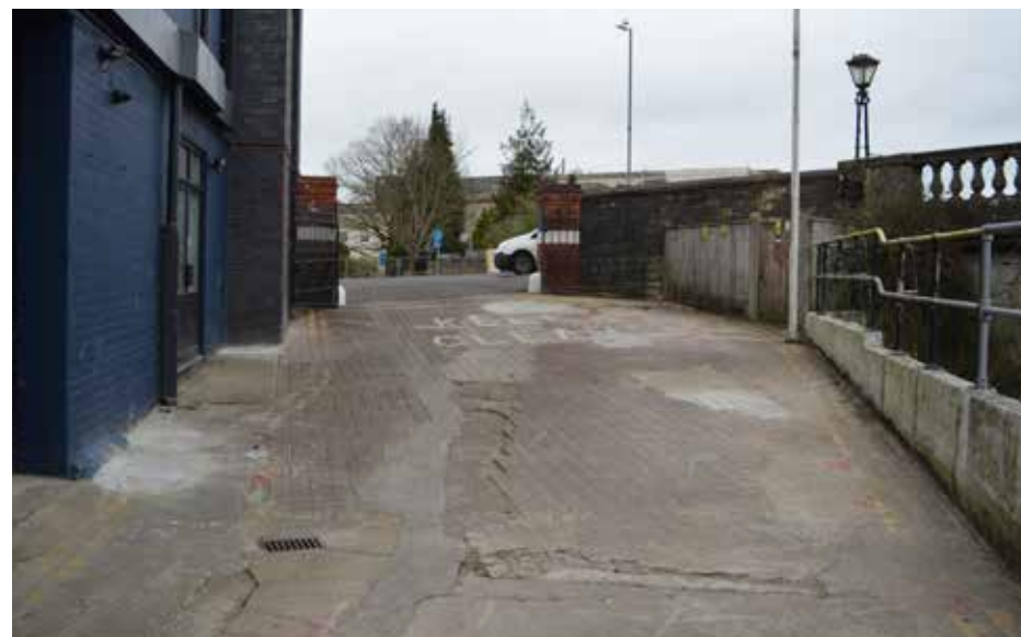
7 - Fractured coloured concrete surface with block paving print
