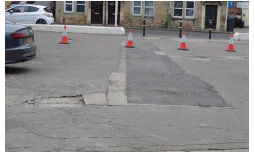
5 - Mix of concrete and tarmac surfaces with localised fractures and repairs
