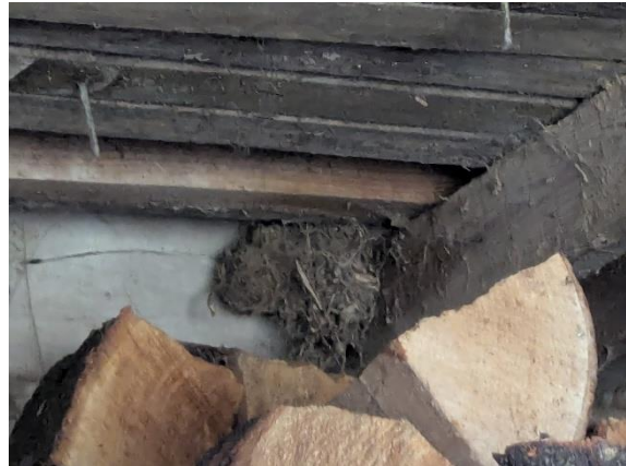
Photo 4 – internal view of field shelter showing example of birds nest found
