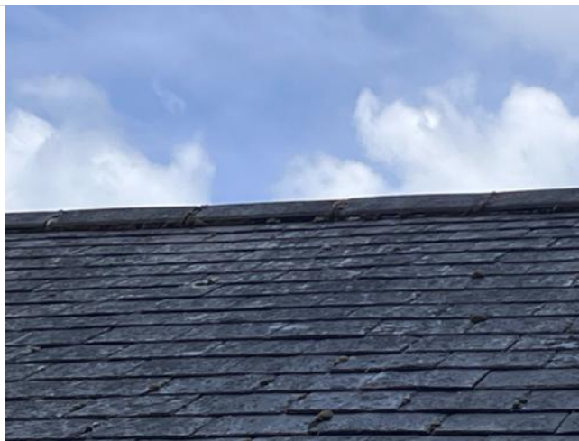
Missing mortar under ridge tiles
