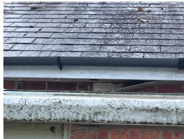
Gaps within soffits
