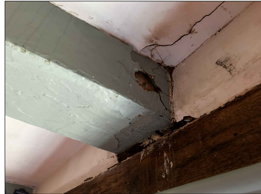
BEAM END SUBJECT TO DAMP CONDITIONS
