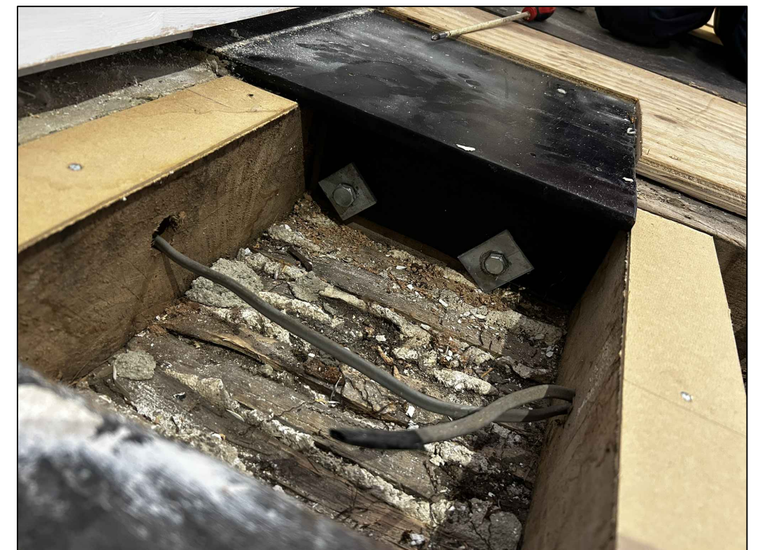
FLOOR OPENED UP WITHIN FIRST FLOOR ROOM. TEMPORARY STEEL BRACKET HAS BEEN INSTALLED BY OTHERS PRIOR TO MLDE INVOLVEMENT. BRACKET HAS BEEN ASSESSED BY MLDE AS INADEQUATE.
