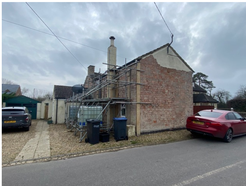
North facing roadside gable with temporary propping to east flank wall 26.01.26
