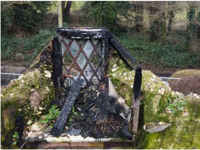
Significant damage to first floor windows and cob walls
