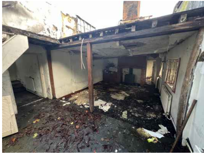
West end first floor failed and collapsed
