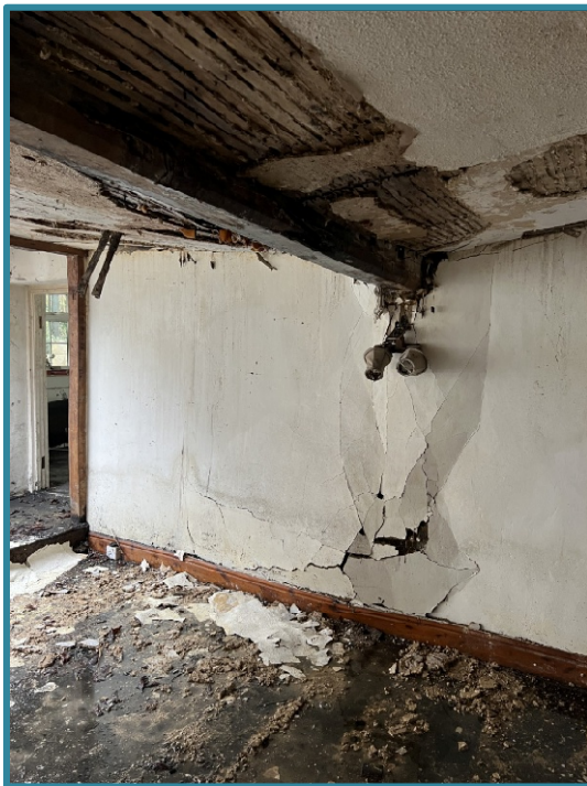
Figure 10 – Failed Bearing in Cob Wall
