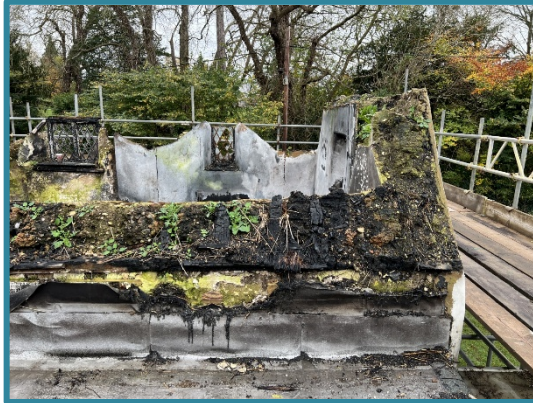
Figure 2 – Charred Remains Roof Timbers
