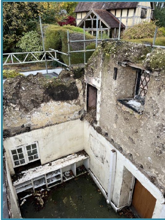
Figure 8 – Exposed Cob to inside of East Gable and North upper Wall
