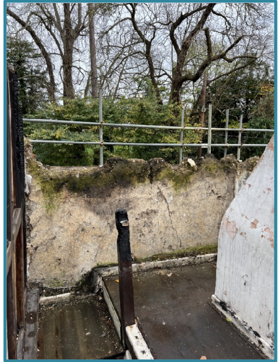
Figure 9 – Fracture to Cob Wall (South Side)
