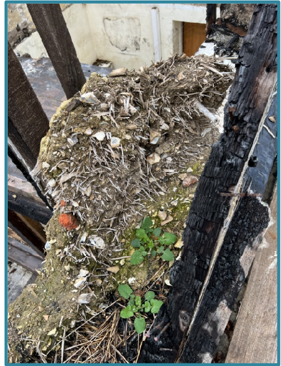
Figure 7 – Badly Weathered Cob
