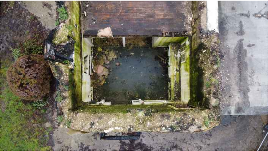
Aerial view of east end, floor lost to fire and significant weathering to cob walls left uncovered
