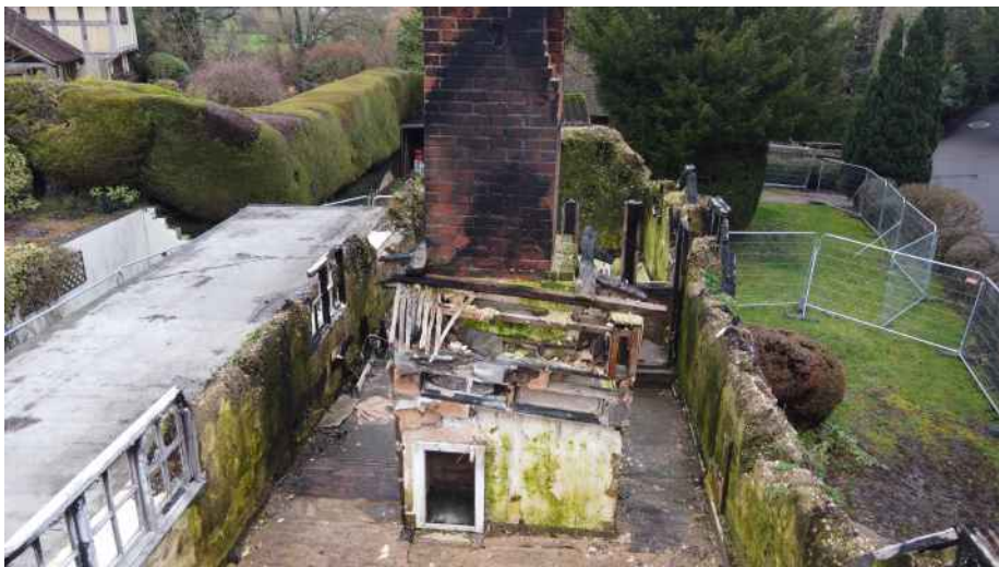
Chimney stack remains, almost complete loss of first floor partition walls
