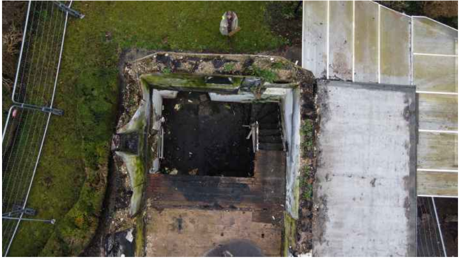
Aerial view of west end, floor lost to fire and significant weathering to cob walls left uncovered
