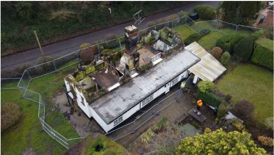
Rear aerial view, significant damage to original house, single storey extension still remains
