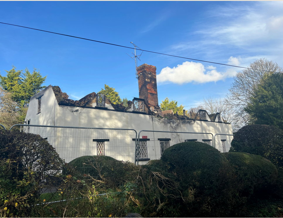
Figure 4 – Hackthorne cottage front elevation, facing North, post fire
