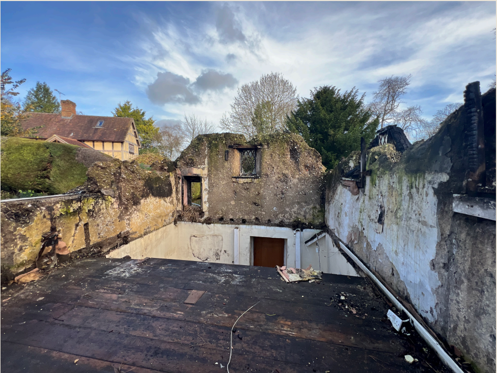
Figure 2 Hackthorne Cottage post fire, collapsed first floor and remains of upper walls
