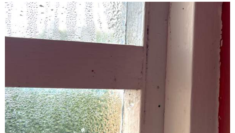
Figure 199 Detail of casement, showing crudely inserted glazing bars.
