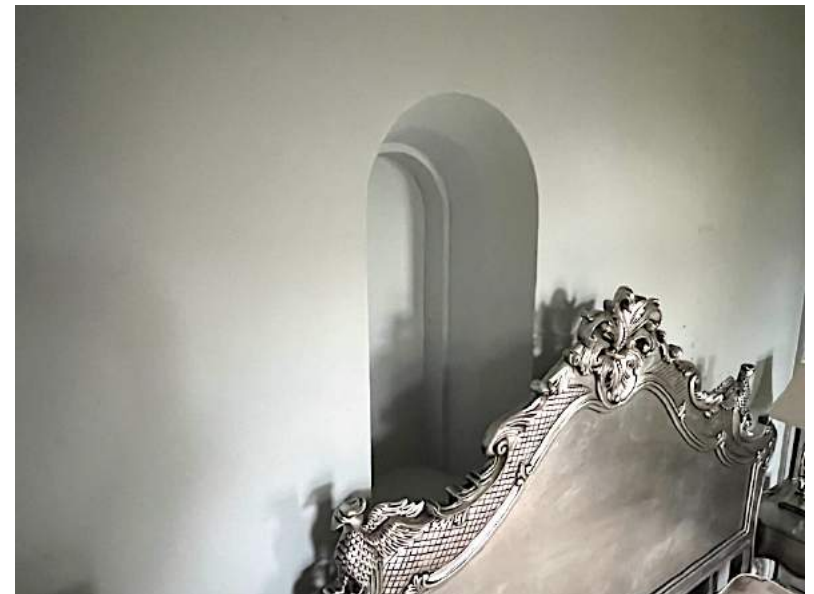
Figure 174 Bedroom (above Gallery ), blocked window on east wall.
