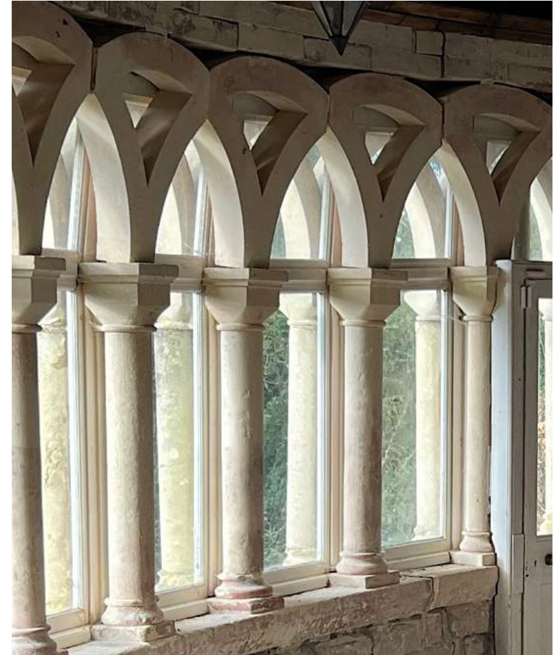
Figure 253 Fernery , detail of arcade showing movement at impost level.
