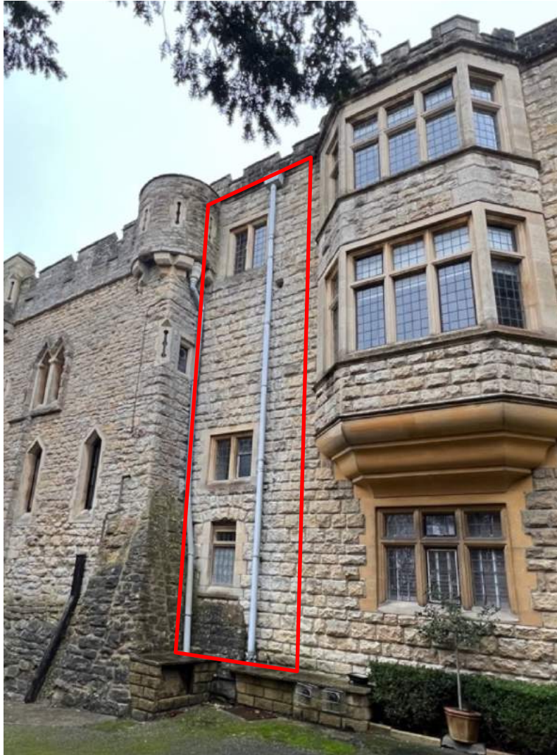
Figure 60 Back stair, external fenestration, showing lower window breaching floor level, but upper window placed normally.
