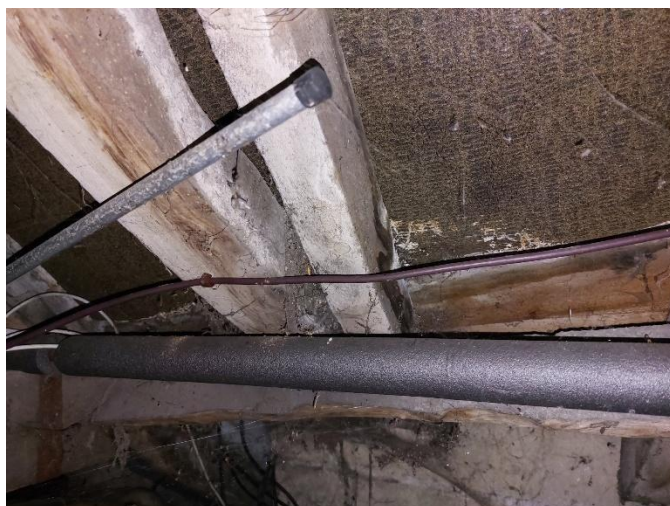
(Roof void from main attic office accommodation with replacement reinforced polythene sheet and older style 1F bitumen felts over old roof structure with some replacement rafters noted, some timber decay noted from water penetration)
