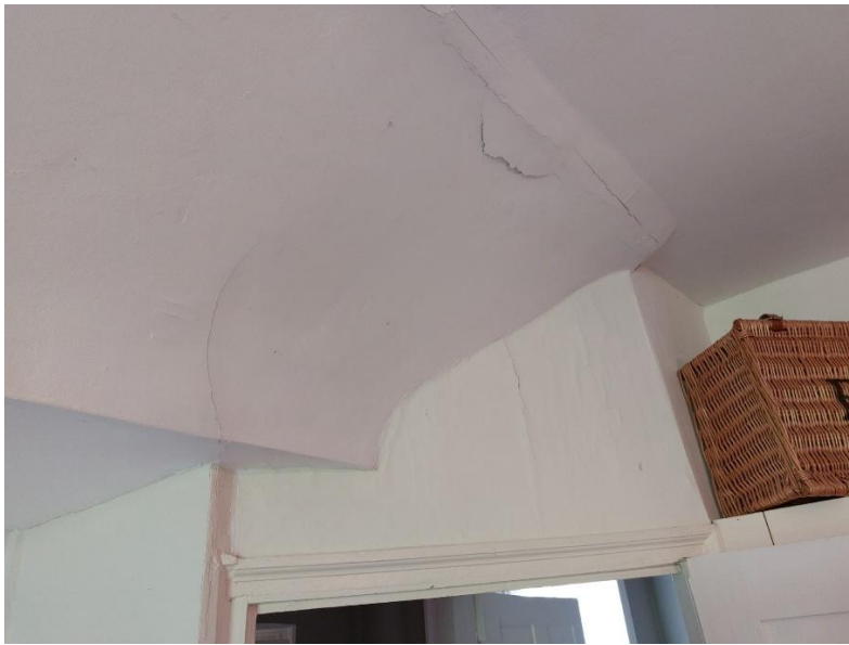
(2 nd floor north west main bedroom, structural movement cracking noted beneath north west gabled roof structure)
