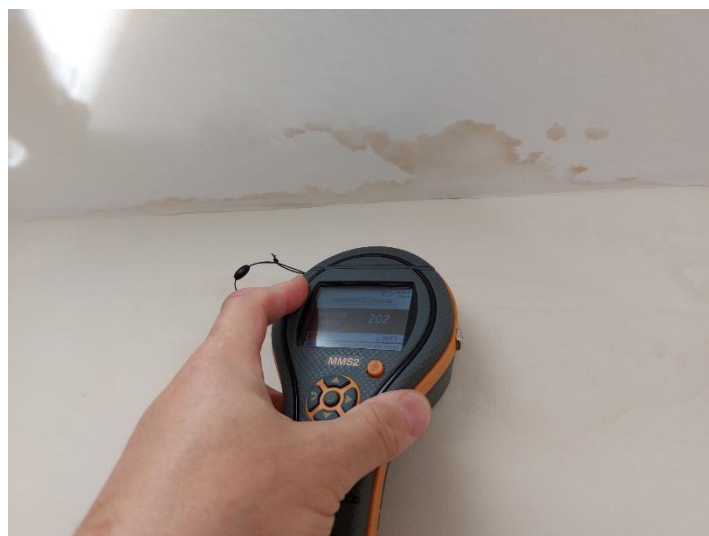
(2 nd floor south east bedroom, cracking and water penetration noted)
