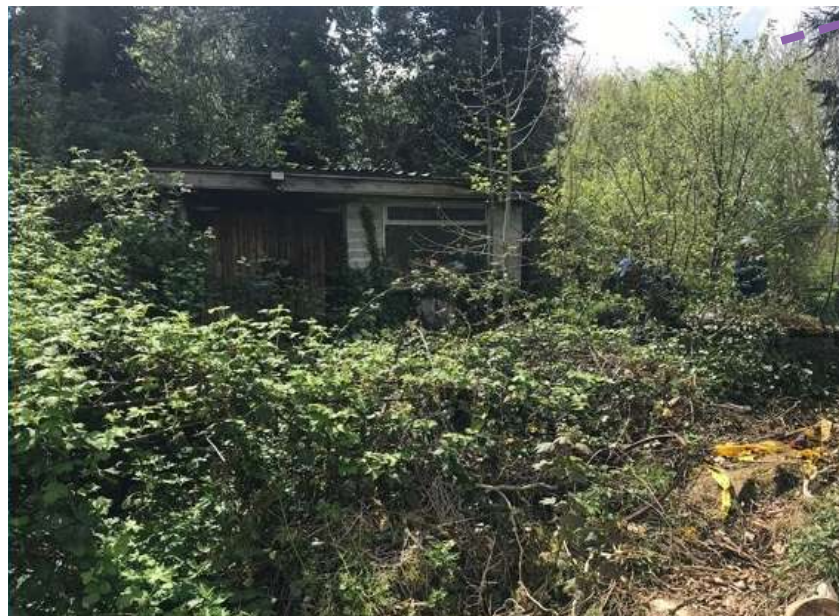
Vegetation completely overgrown. Outbuilding in dangerous state of disrepair. Unable to access tall trees which required urgent management.
